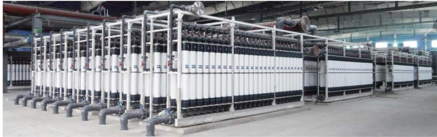
Ultrafiltration membrane modules factory of 20m 3 /d reclaimed water plant
